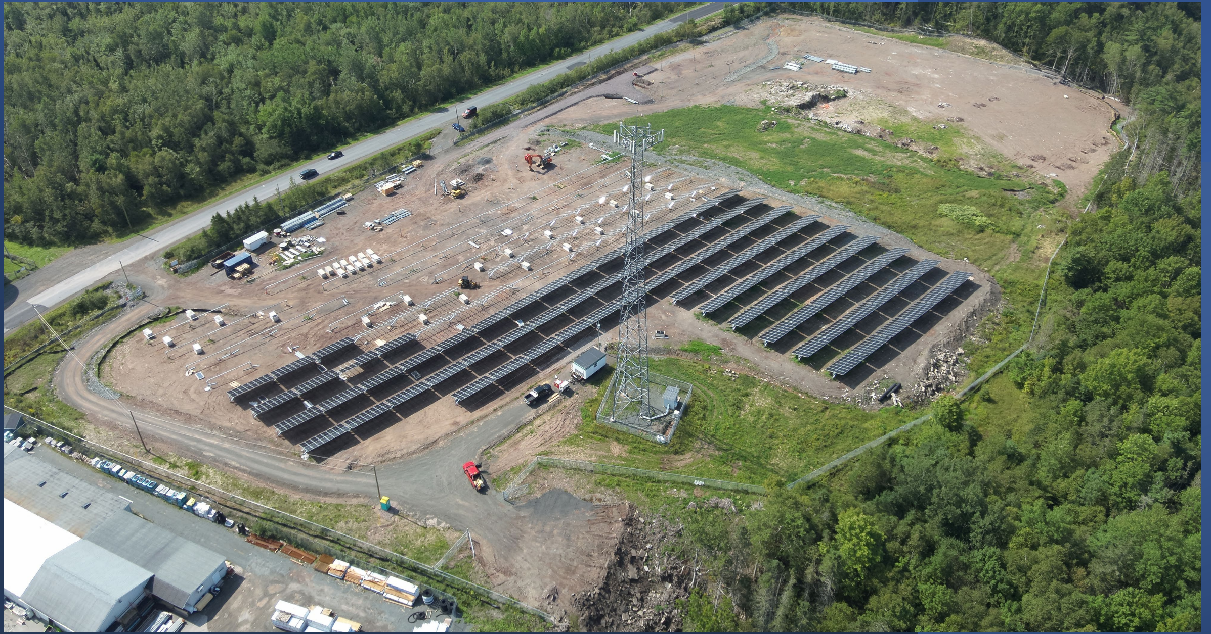
Town of Antigonish 1.65 MW Solar Garden
